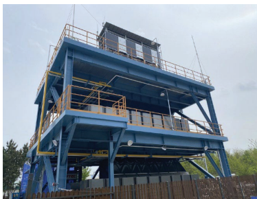
Figure 3: 1.8 MW Power Tower with Heat Capture Installation (3x600 kW)
